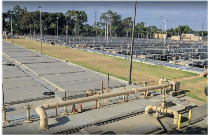
Figure 6.1: Los Coyotes Water Reclamation Plant
